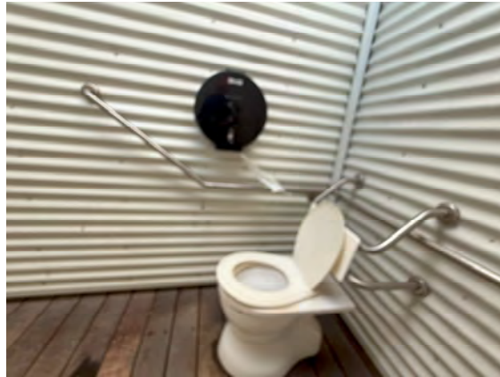
Figure 20: "Accessible" toilet at (a) Ocean Grove unsealed carpark bridge
