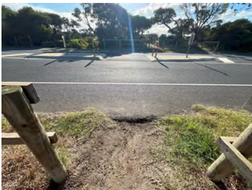
Figure 12: (a) No warning kerb to roadway
